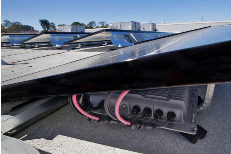
Figure 2: Clearly identified string polarities make miswiring harder
